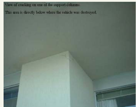
View of cracking on one of the support columns. This area is directly below where the vehicle was destroyed.
