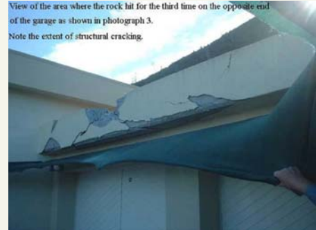
View of the area where the rock hit for the third time. Note the effect of structural cracking
