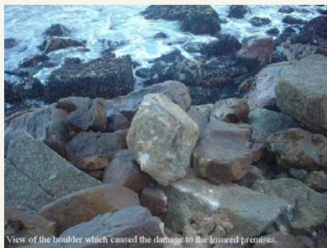
View of the boulder that causes the damaged to the insured premises.
