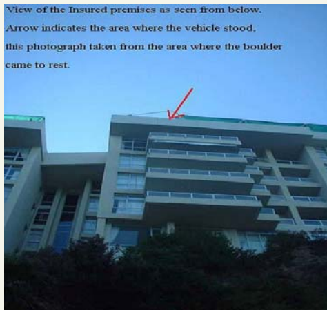
View of the insured premises from where the boulder came to rest. The arrow indicates where the vehicle stood.
