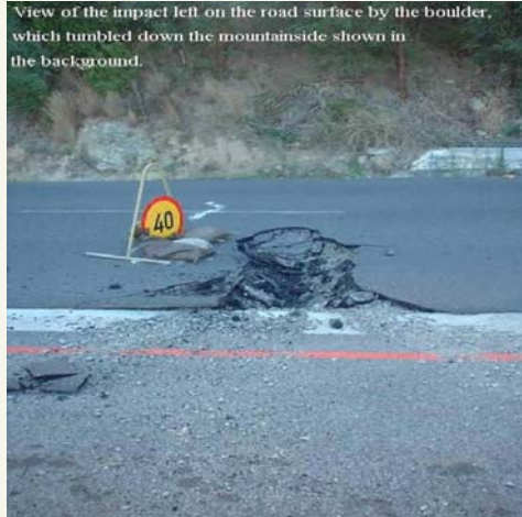
View of the road surface damage from a boulder that tumbled down the mountainside
